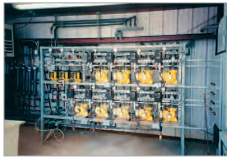
Coagulant / Polymer / Acid Feed System with Dilution Water
