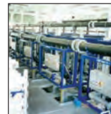
Bedok Water Reclamation Site, Singapore Reclaiming 3.4 MGD (13,000 m3/day)
