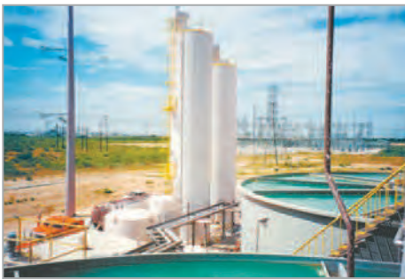
Lime / Soda Ash Storage
