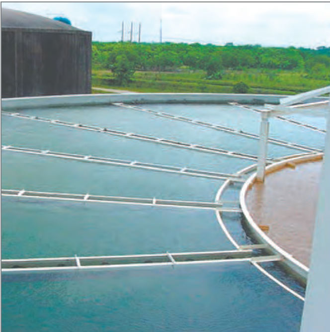
Surface Water Clarification
